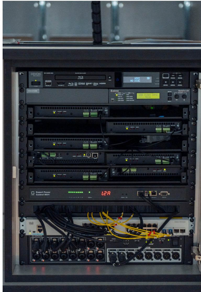
Expert Power Control 8031-1 controls and monitors the power supply in the 19-inch rack in the lecture hall desk Photo: © University of Siegen
