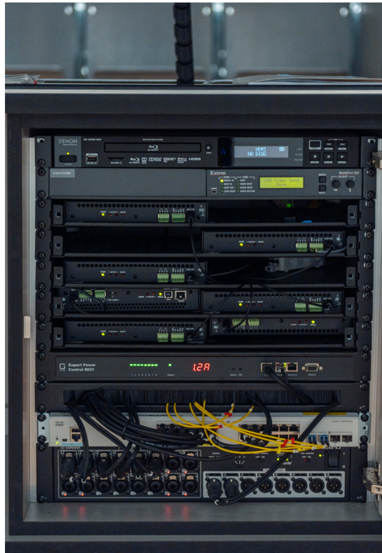
Expert Power Control 8031-1 controls and monitors the power supply in the 19-inch rack in the lecture hall desk Photo: © University of Siegen
